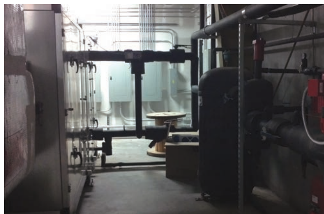
High Purity Standards mechanical room.
